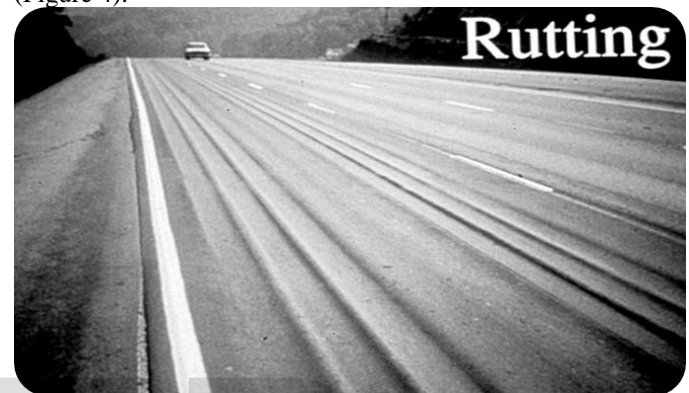
Figure (4) Rutting is apparent in the wheelpaths of this street
